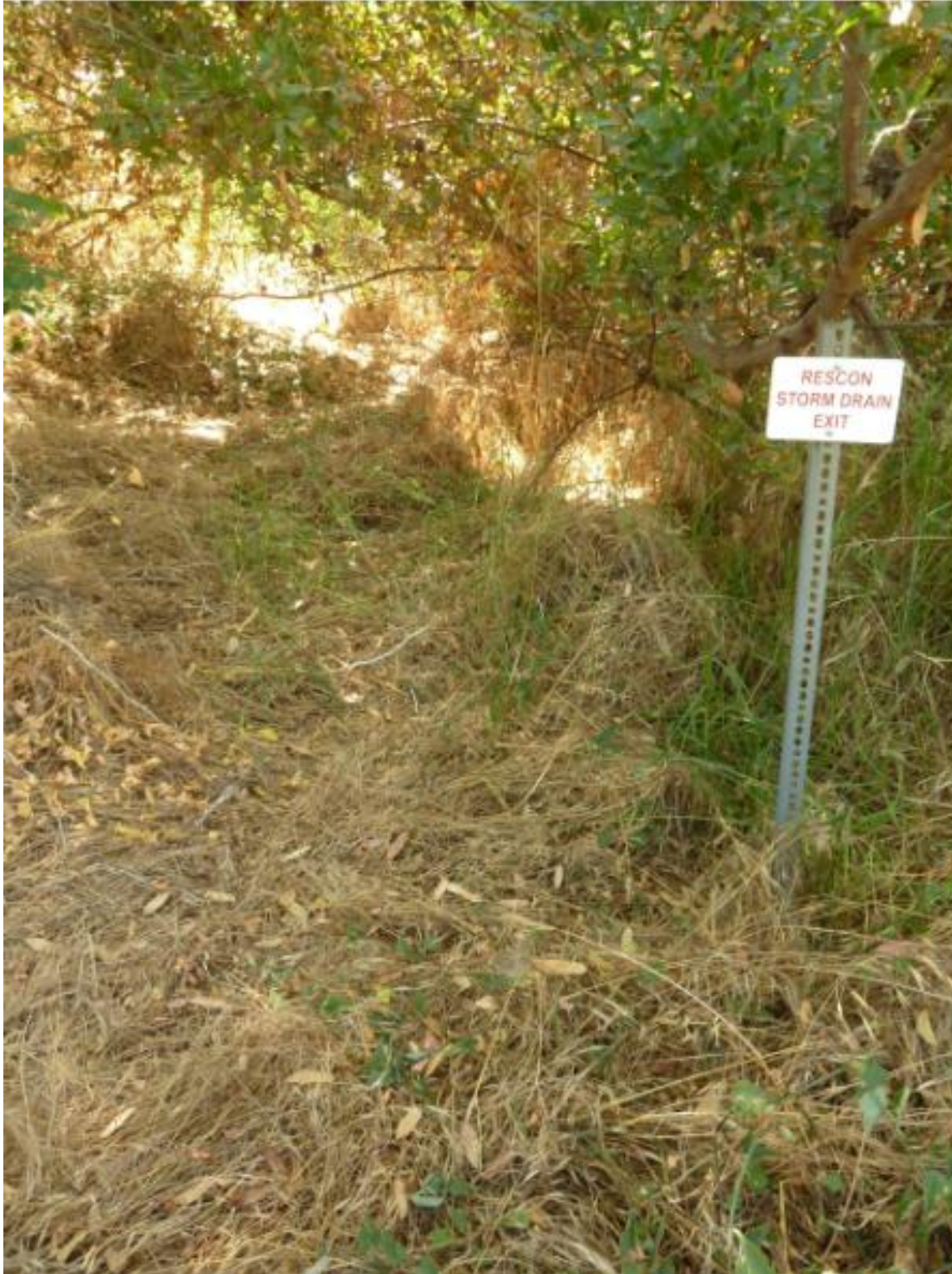
Figure 2. Storm drain exit on the south side of the Park road leading to a private residence. Runoff from this storm drain should be re-directed to the other side of the road so it will drain into Drainage Basin E instead of Basin G.
