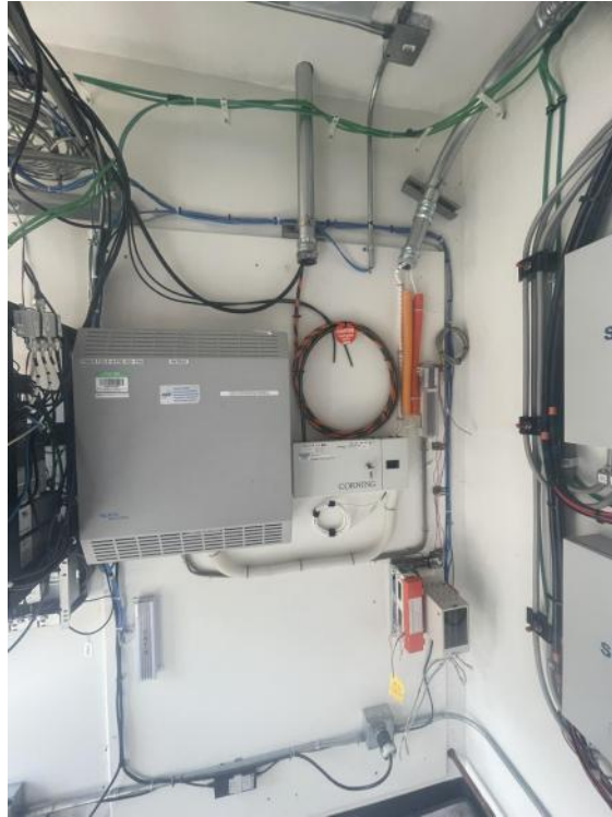
AC Unit Controls
