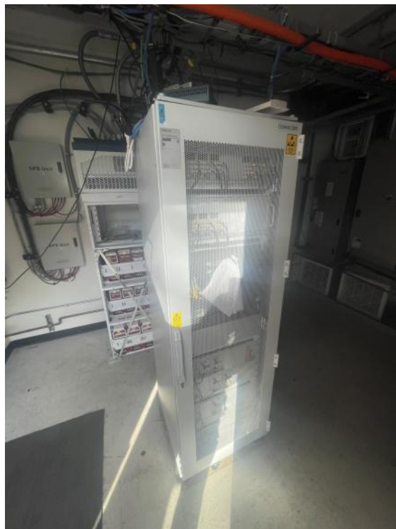
View Inside Shelter
