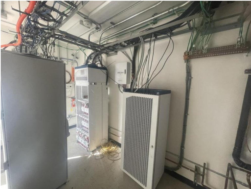
View Inside Shelter
