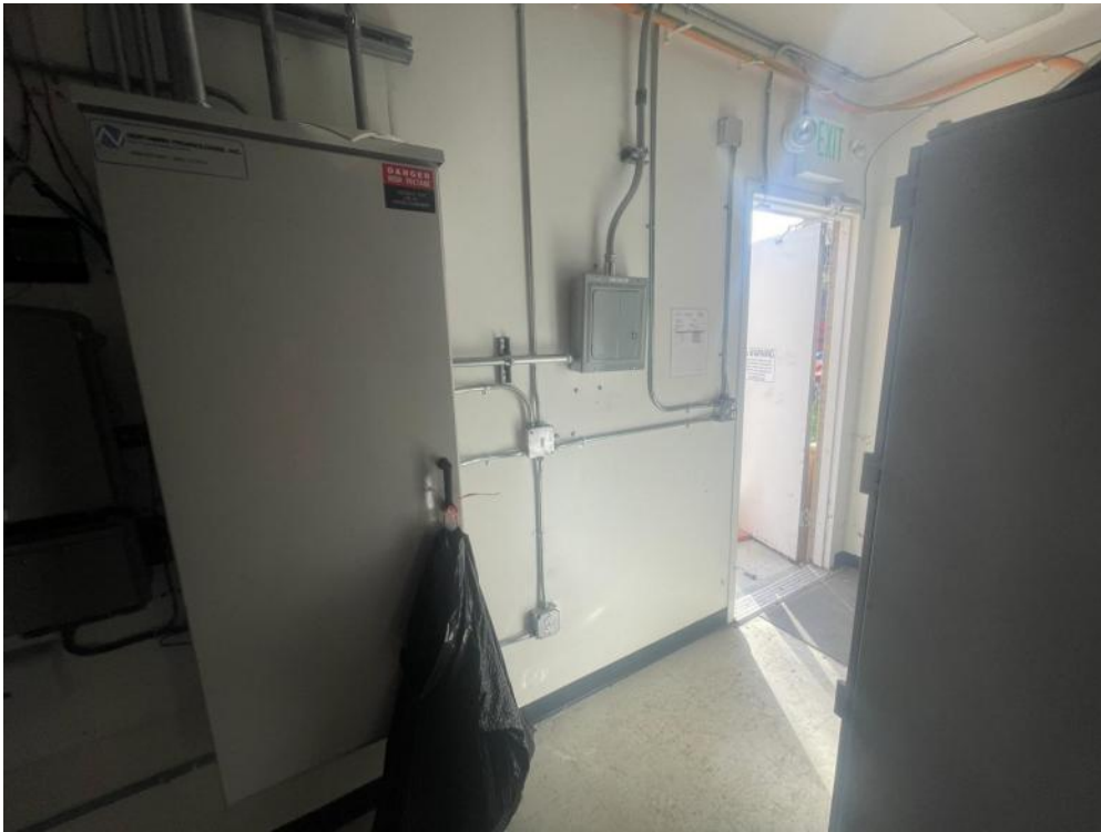
View Inside Shelter
