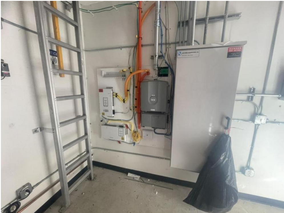
View Inside Shelter
