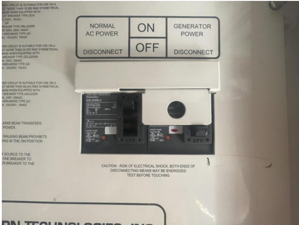
PPC Main 200A Breaker
