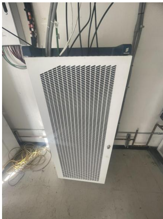
BTS Equipment Cabinet
