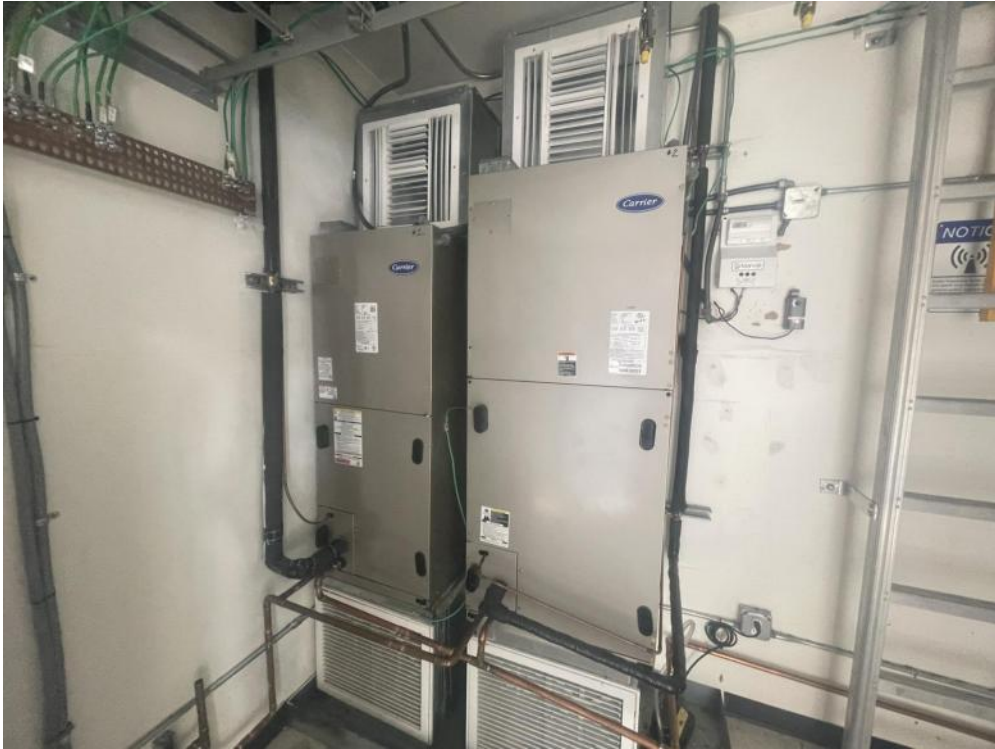
View Inside Shelter
