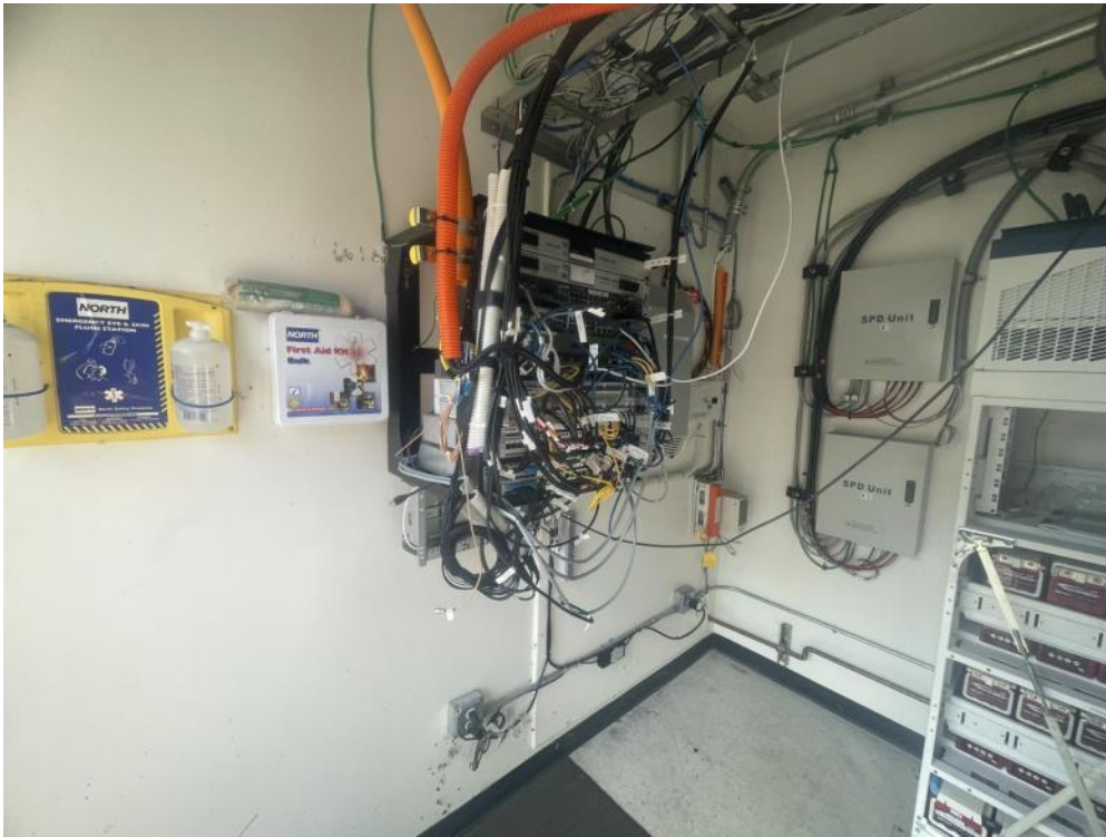
View Inside Shelter
