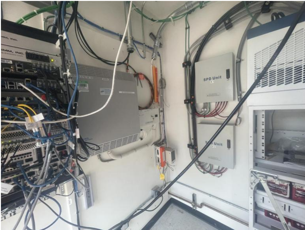
View Inside Shelter
