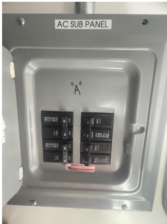
AC Subpanel Breakers
